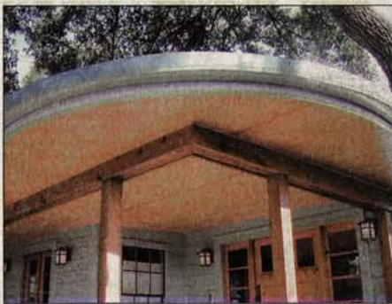
The front entry porch at West 41st Street interweaves colors and materials to mimic the outdoor landscaping in an eclectic design.
